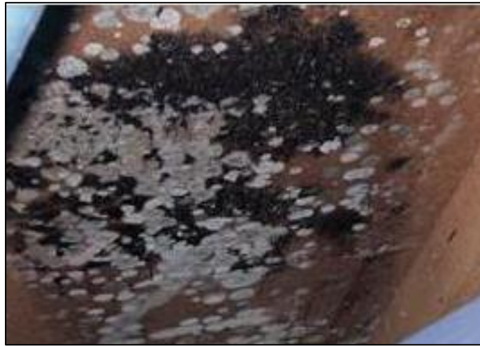
Figure 4.12 Interstitial condensation resulting in mould through a wall.
