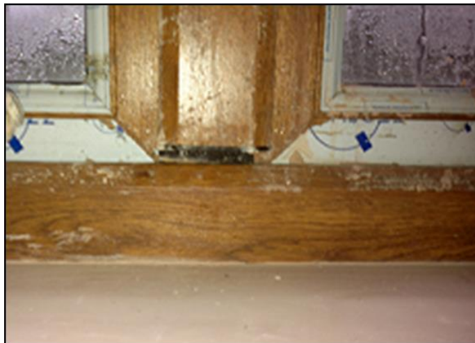
Figure 4.11 Surface Condensation on windows
