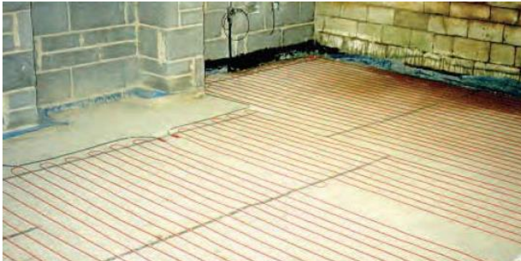
Figure 4.5 Electric underfloor heating elements prior to receiving a layer of screed (Source www.bsria.co.uk )
